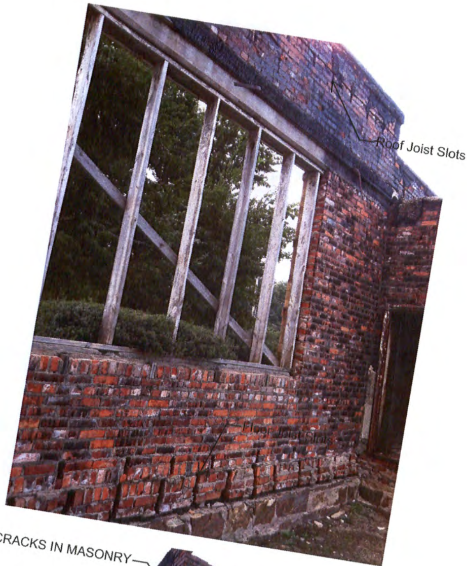
PICTURE 1 Shows Existing Masonry Wall where the floor diaphragm and roof diaphragm were connected.
