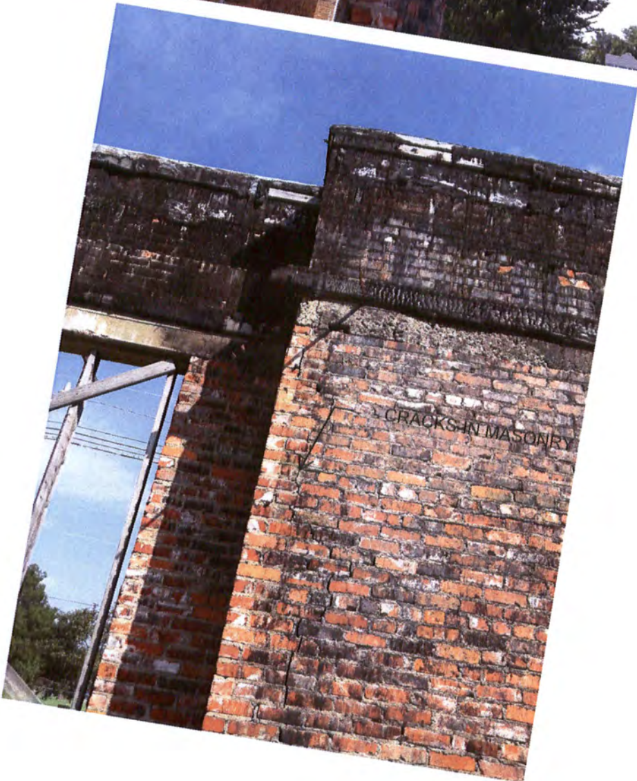
PICTURE 4 Shows Cracks in the Existing Masonry Wall.
